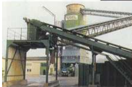
GREASE MAX ® installed at a Quarry
